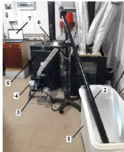
FIGURE 3. Experimental installation of a pellet burner for burning vegetable pellets: 1 – loading hopper; 2 – external auger for transportation of biofuel; 3 – pellet burner; 4 – fan; 5 – solid fuel boiler; 6 – boiler control unit; 7 – unit of measurement and archiving of experimental data
